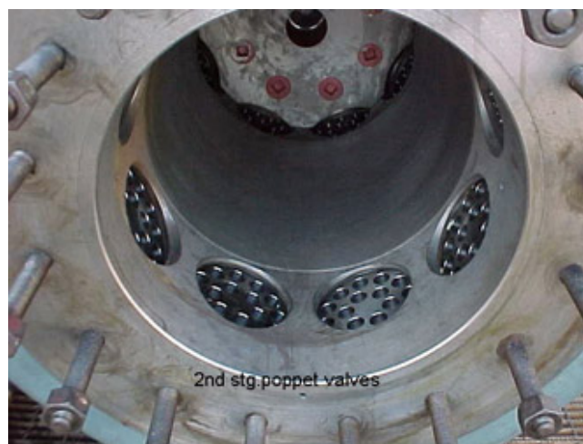
Figure 2.1: Working chamber with removed cylinder head
